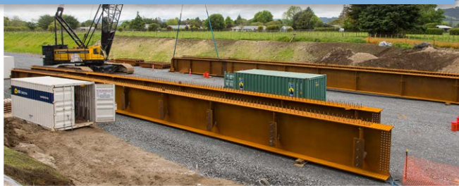
Steel beams ready for placement The cargo containers give a sense of how massive each beam is.
